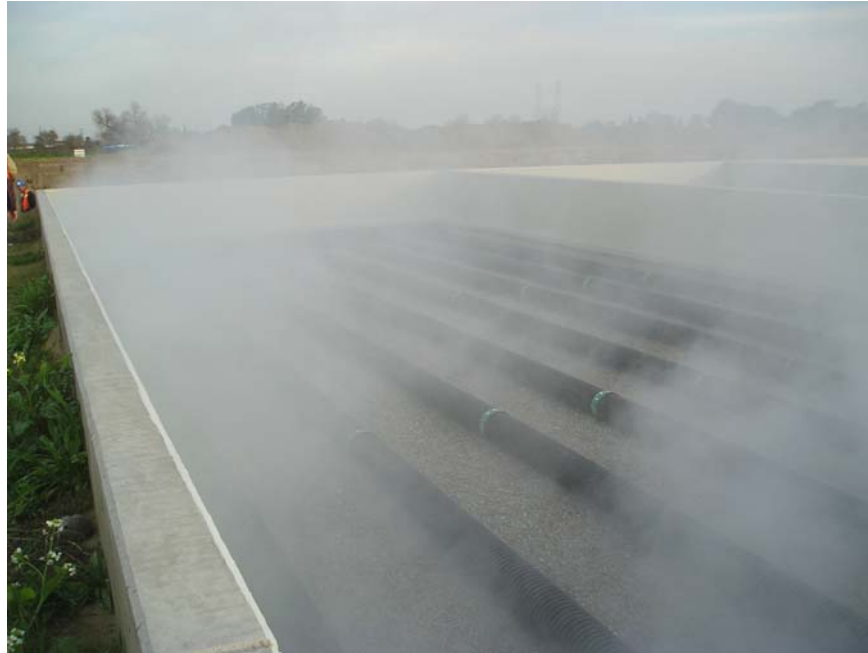
Figure 5 – First Smoke Test in a Biofilter Bed
